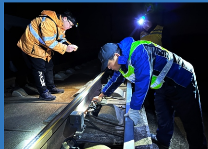
Sensor on-site installation
